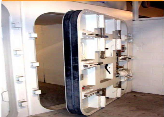
Tunnel Flood Door
