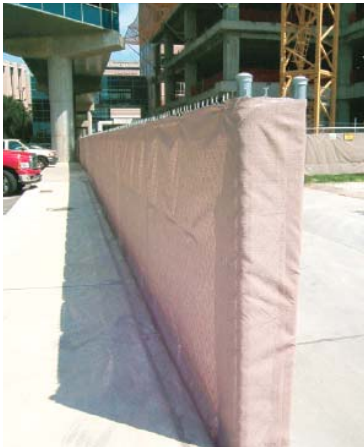
Perimeter fencing in accordance with TMC specifications
