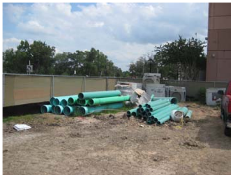
Building materials need to be removed or secured
